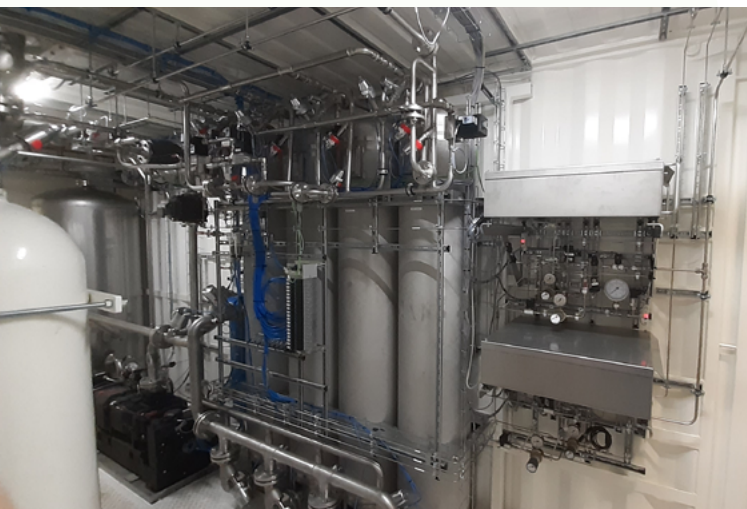
Figure 6: PSA unit. Credit: Fraunhofer UMSICHT.
